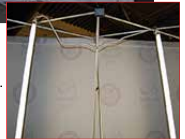
Link cable connection close up.
